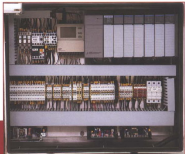
▲ Centralized electrical panel control
